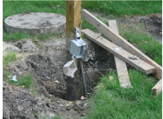
Flood damaged SSTS electrical box
