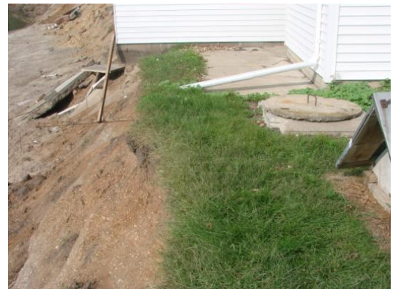
Washed away SSTS in eroded stream bank
